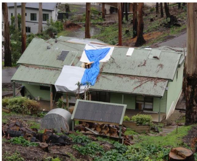
Figure 3: A house on Wallace Street, Wye River damaged by tree strike caused by fire.
