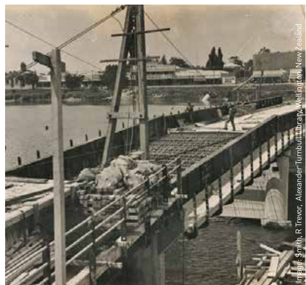
Wairoa River Bridge, Wairoa, Hawke's Bay, under repair after the 1931 Hawke's Bay earthquake.
