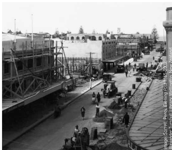
Men working on the road and buildings in Emerson Street, Napier, after the earthquake of 1931.
