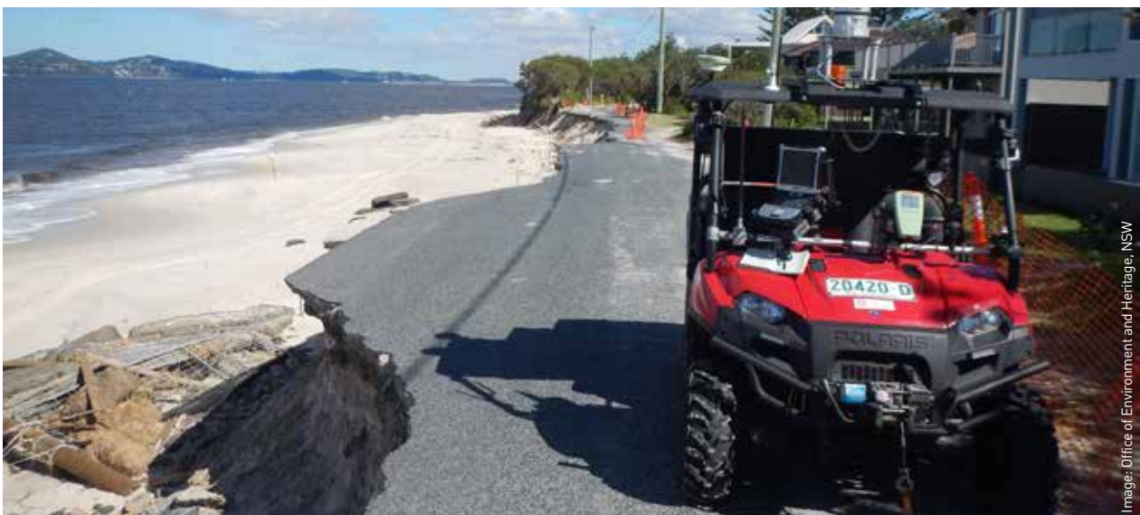
The Office of Environment and Heritage NSW assess erosion at Jimmy's Beach, NSW, after storm damage in April 2015.
