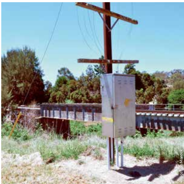
Molong Railway Bridge showing estimated flood height on the electrical box.
