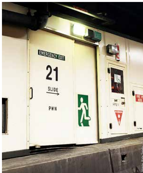
Impediments to evacuation. The jersey barriers had two small cut away steps (visible in bottom right of this photo) which the elderly participants were unable to use without assistance. They took around five seconds to climb the barriers with assistance.
