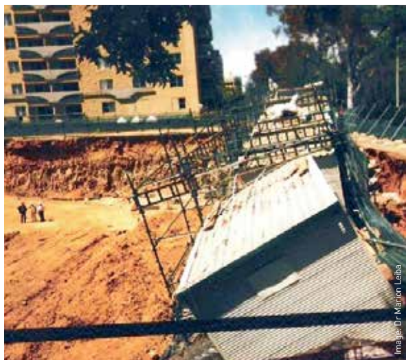
A landslide at a building site in Canberra causes two prefabricated site buildings to come off their foundations.
