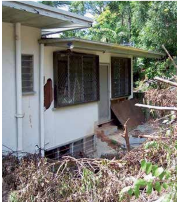
Fill failure in a disused road inundates a house in Cairns.
