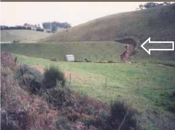
FIGURE 5. Dam No. 6 in 1995 showing the spillway undercutting and weakening the dam wall. The embankment was otherwise well maintained.
