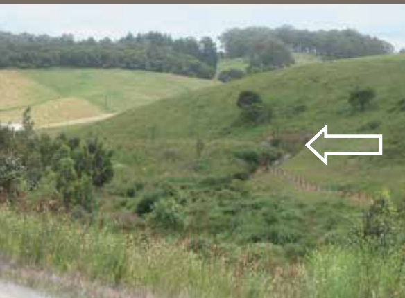
FIGURE 6. Dam No. 6 in 2007 showing the spillway still undercutting the dam wall. Dense vegetation is also now allowed to grow out of the embankment and to completely block the spillway.
