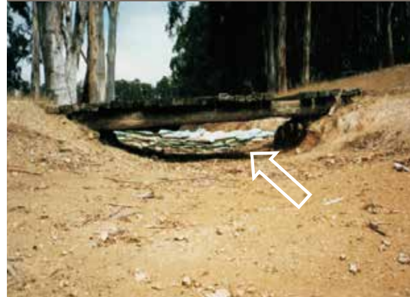
FIGURE 1. Dam No.2 in 1995 showing the spillway blocked by a walk-way bridge and sand bags, and trees allowed to grow out of the crest.
