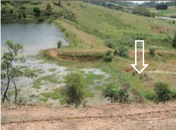
FIGURE 4. Dam No. 4 in 2007 showing the spillway still blocked by a mound of dirt, but now shrubs and vegetation are growing in the spillway and along the upstream face of the embankment.
