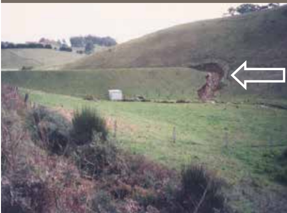
FIGURE 5. Dam No. 6 in 1995 showing the spillway undercutting and weakening the dam wall. The embankment was otherwise well maintained.
