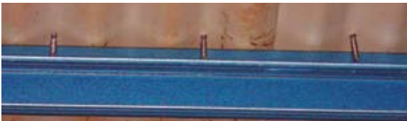
Figure 9: Roofing screws missed top hat batten.
