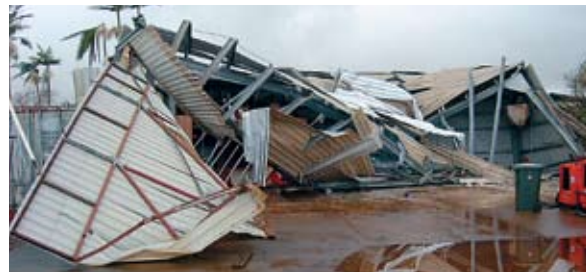
Figure 7: Failure of cold formed steel frame shed
