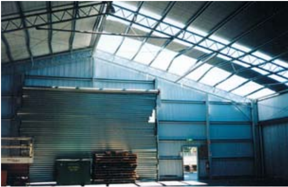
Figure 9: Structural failure of shed from failure of roller door on windward wall
