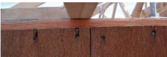
Figure 10: Gun nails over driven in bracing panel.
