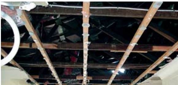
Figure 8: Ceiling damaged by water ingress from debris impact to gable
