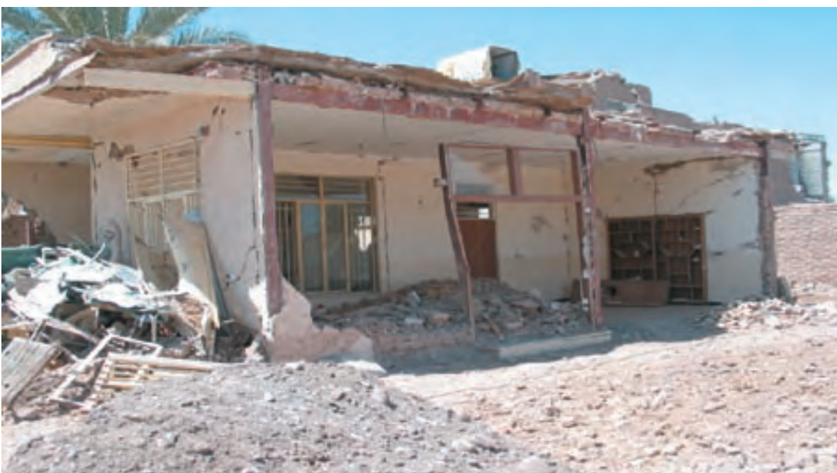
Fig 5: Damaged houses such as this one were classified on a grading system from 1-5.
