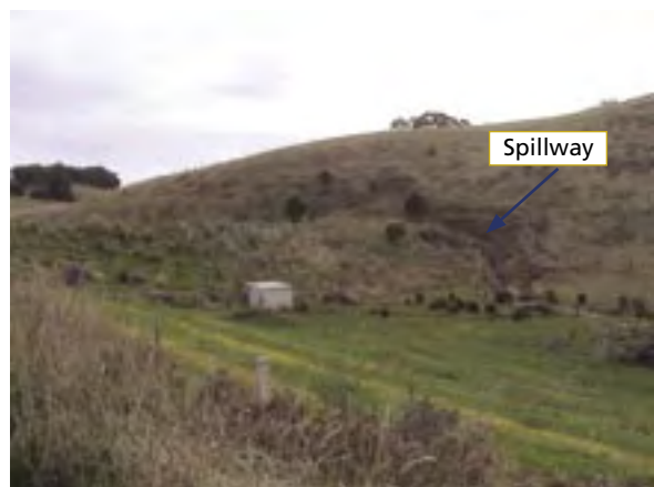
A poorly designed spillway as it undercuts and weakens the dam wall: the potential exists for the wall to collapse at any time, particularly during a significant overflow event.
