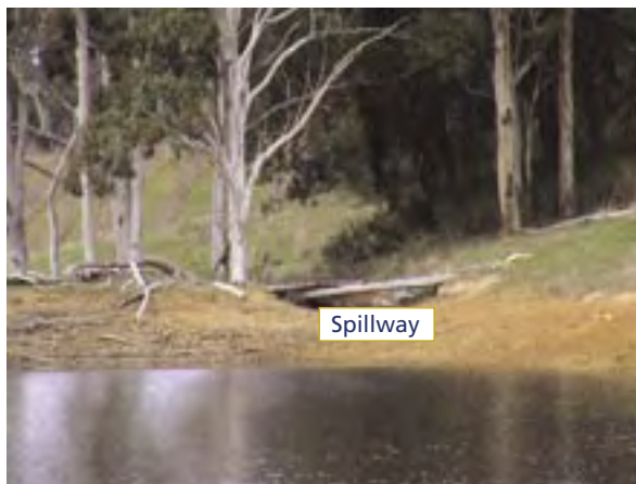
An under-designed spillway; its size is clearly too small for this 100 ML impoundment. The spillway is also badly maintained as the owner allows physical obstructions, including a walkway bridge and sandbags, to be present across the spillway restricting its potential capacity.
