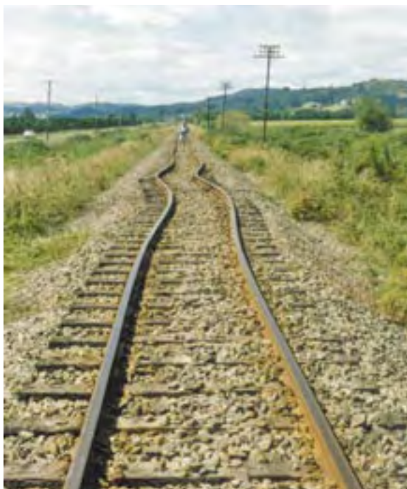
Travel disruptions and freight transport can be disrupted by rail lines buckled by earthquake
