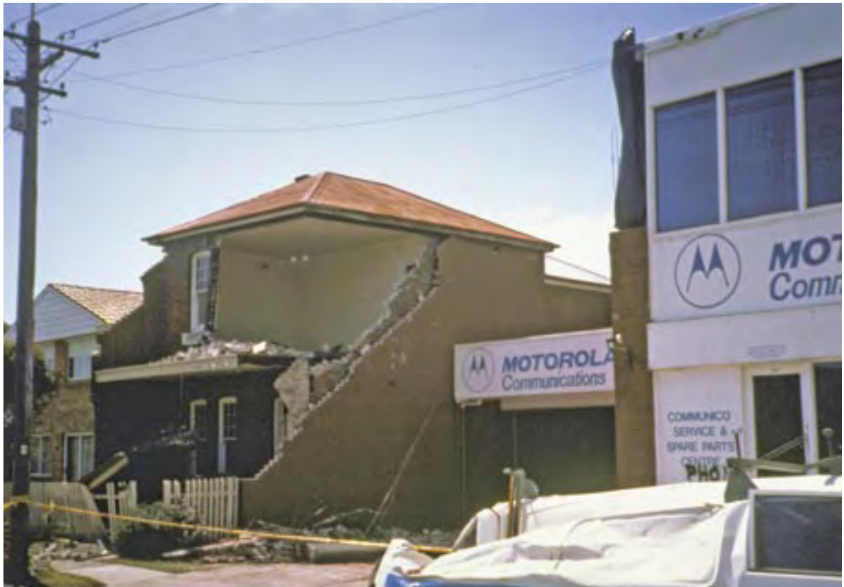
While the house at the centre of the photograph has been damaged, those around it have remained relatively intact. Differences in quality of construction or maintenance can help explain the uneven distribution of damage. This highlights the importance of including building checks and regular maintenance in an earthquake preparedness plan and rectifying any problems to minimise damage
