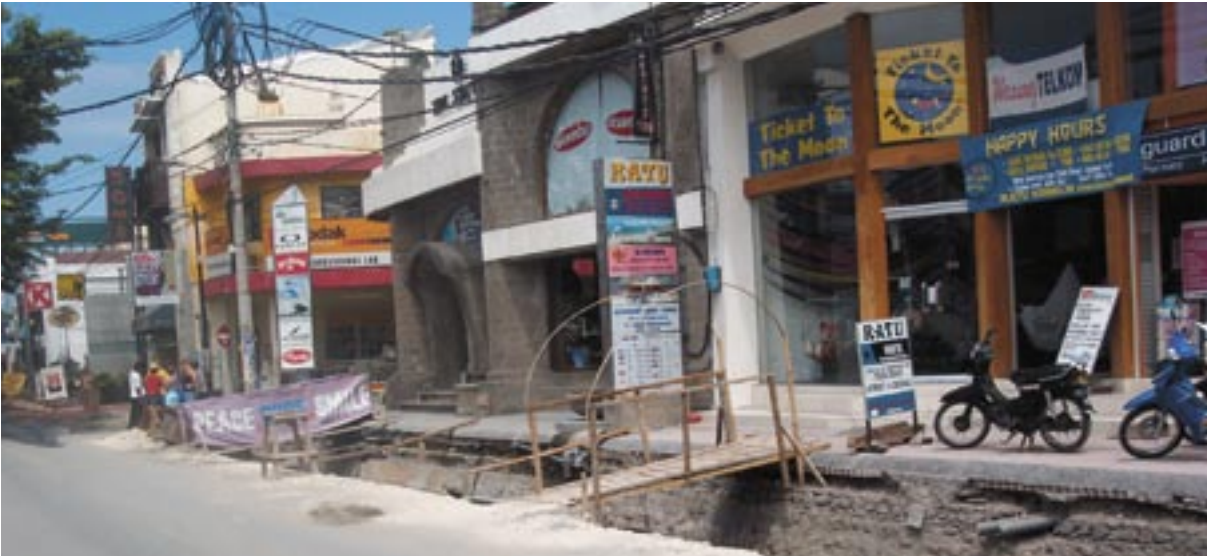
Over the rubble of destroyed buildings on Legian Street many tourism businesses are rebuilt
