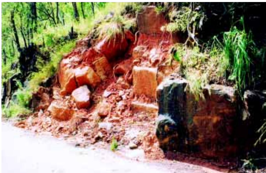
This small landslide on the Paluma Road, north of Townsville, killed a woms during Tropical Cyclone Justin in March 1997
