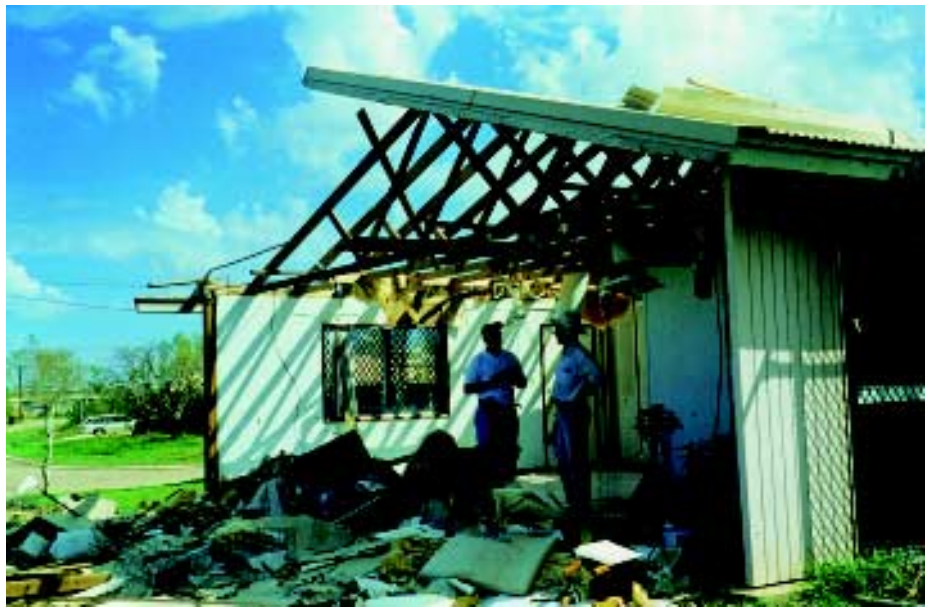
Photo 5: Failure of the end wall due to interior pressurisation.
