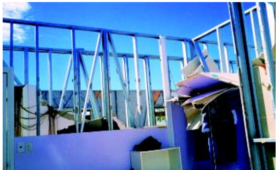
Photo 3: This new transportable home lost its entire roof structure due to inadequate fixing of trusses.
